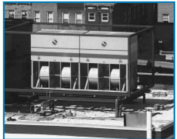
Series V Cooling Tower installation in residential area.
